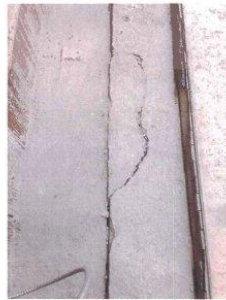
Photo 26: Floor Crack at Room 12
