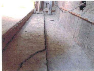
Photo 25: Floor Crack at Room 12
